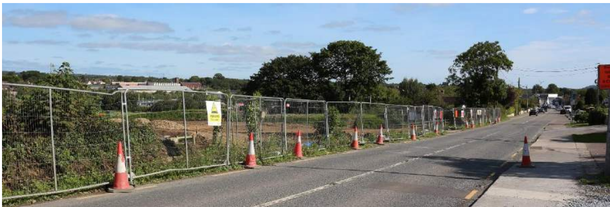
Figure 10-7: Plate 10.5 View eastward along Kilmoney Road Lower showing works associated Western Relief Road
