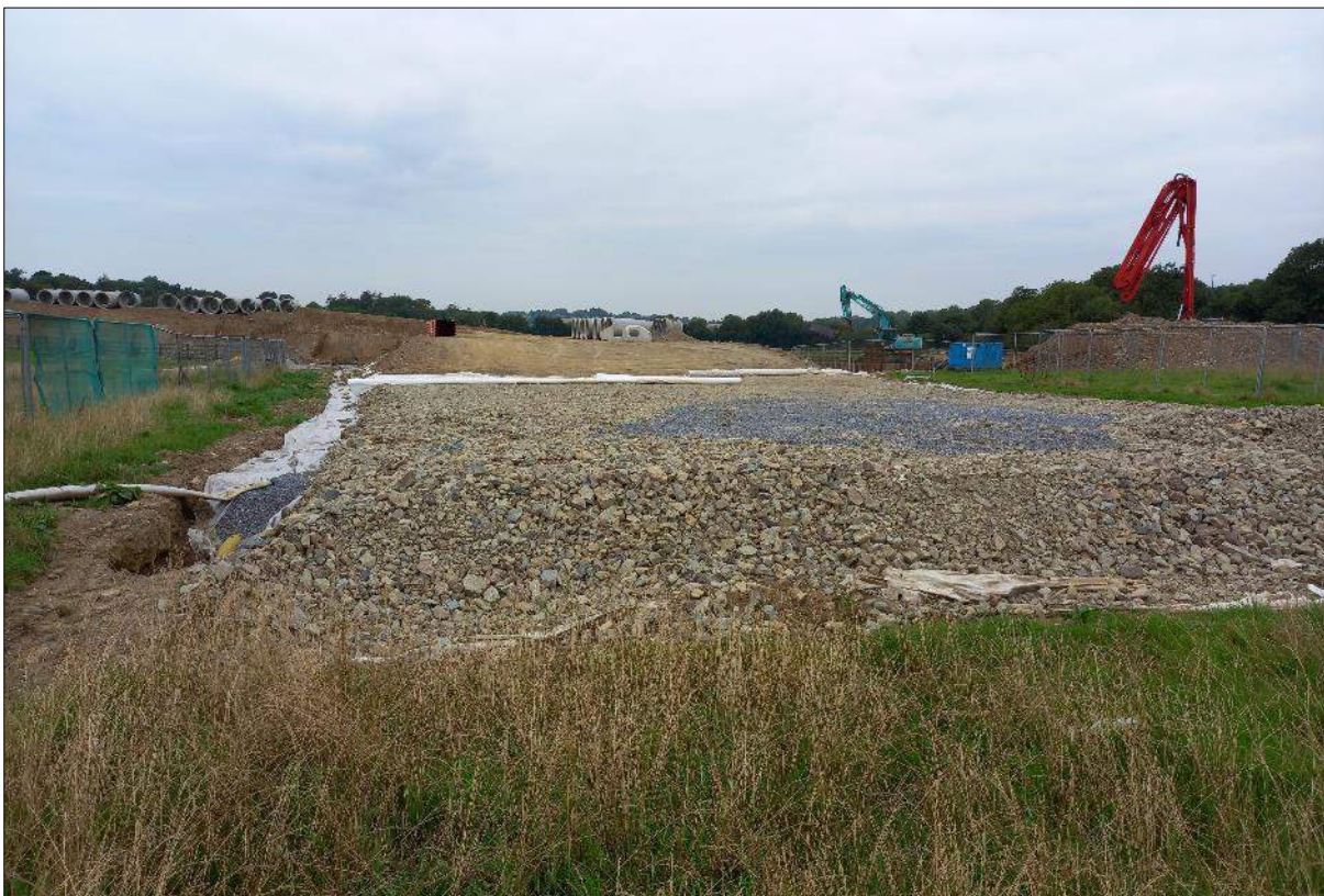
Plate 11.10: View of the hardstanding area constructed within the SHD boundary during the Relief Road works. This is the area of the feature noted on aerial imagery of the site
