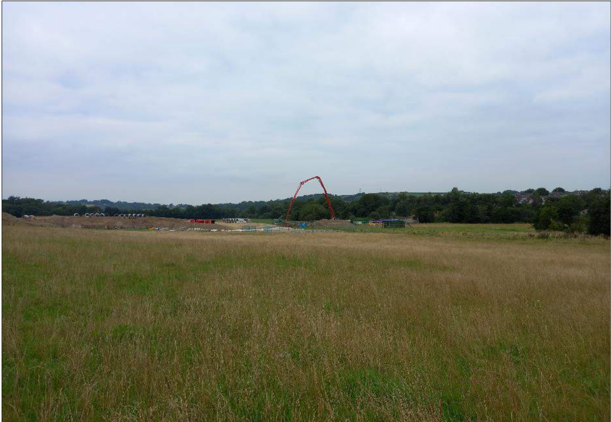
Plate 11.5: View westwards across Proposed Development Site towards the Relief Road which is under construction
